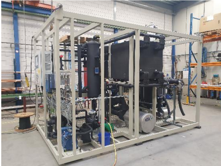
Freeze concentration installation
